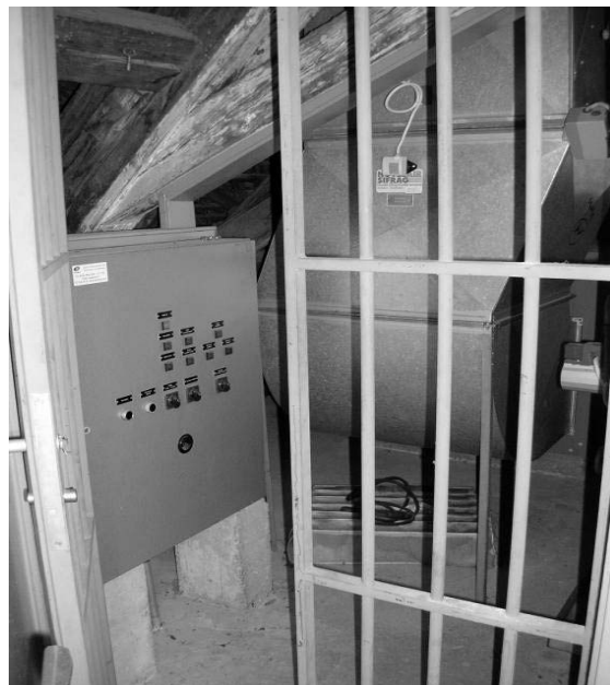
Installation technique - local de ventilation aux combles
