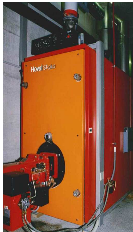
Installation de chauffage existante
